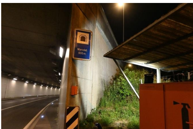
CuGa1 Left wing wall Axis 1 1216 other cracks Close to rubber gasket. Scattered cracks.
