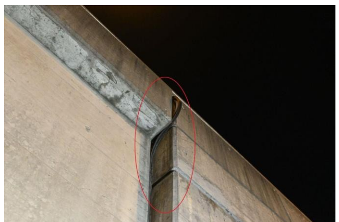
CuDr1 Wing wall Right Axis 1 1209 Joint cracks Upper part of the infrastructure object. The rubber is partially torn off.
