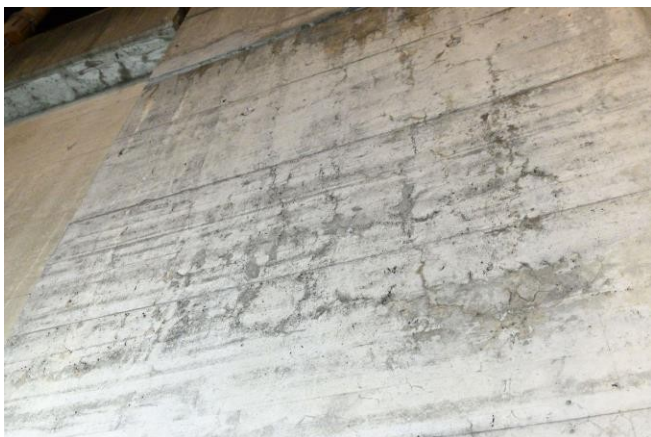
CuDr1 Wing wall Right Axis 1 1303 Eclats At the center of the infrastructure object. Concrete spalling and cracking.
