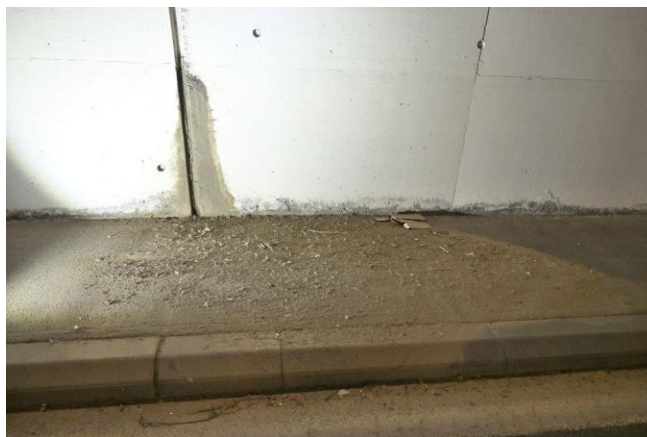
CuDr Straight Cillwall 301 Wetlands Lower part of wall (150m N). Leaky joint, causing seepage.
