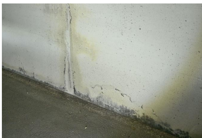
CuGa Culée Wall Left 301 Wetlands Over the entire height of the wall (140m N). Infiltration weakening the concrete.
