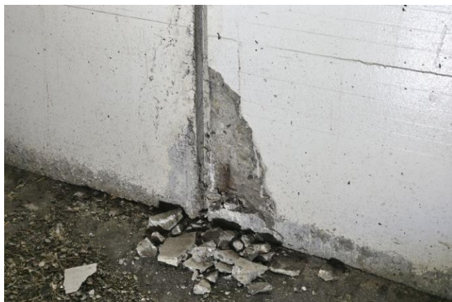
CuGa Culée Wall Left 1303 Eclats Lower part of the wall (25m N). Shattering of the coating.
