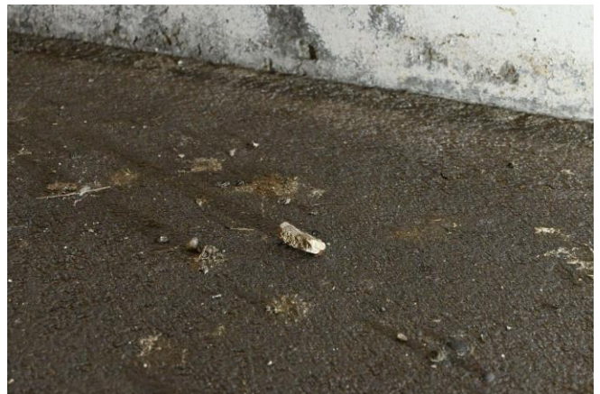
CuDr Straight Cillwall 301 Wetlands Pipe zone - Axis 1 exit (3m N). Concrete spalling and seepage.
