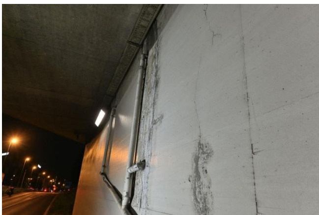
CuDr Straight Cillwall 301 Wetlands Piping zone - Axis 1 exit (3m N). Concrete spalling and seepage.
