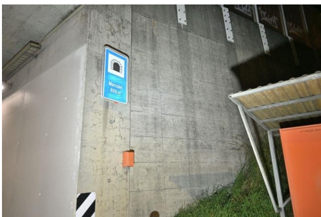
CuDr0 Wing wall Straight Axis 0 1216 other cracks Front face of gate. Surface microcracks.
