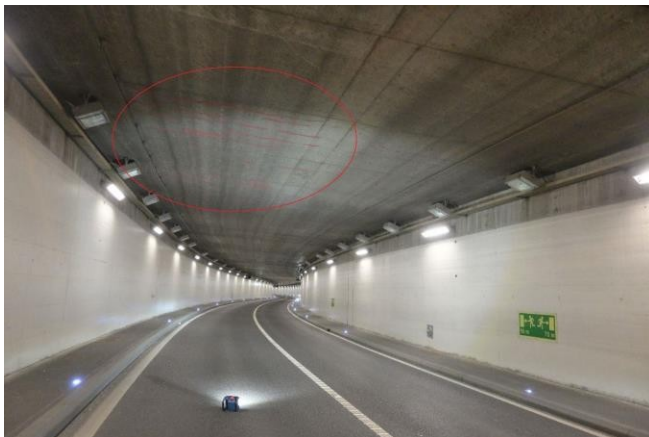
Da Dalle 1216 other cracks Above the track on the right (70m N). Microcracks marked with red spray.
