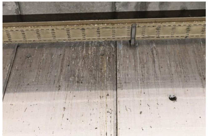
CuGa Culée Wall Left 309 Fouling Upper part of the wall (50m N). Bird droppings.
