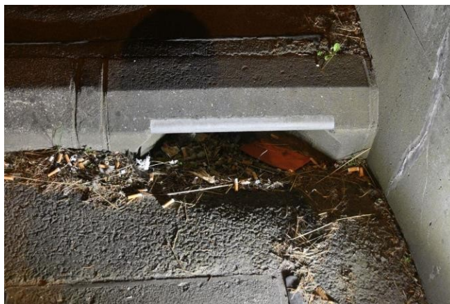
Bo Bordure 411 Malfunctions Drain near left edge of Axis 1. Drain partially blocked by garbage.
